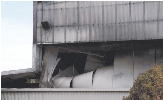
EPS panels at a poultry processing facility fire in Australia, January 2010.
