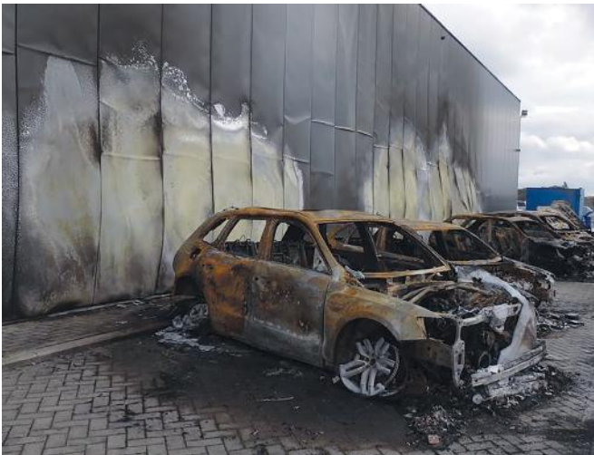
Kingspan Insurer Certified PIR panels at a car dealership in Belgium, October 2014.
